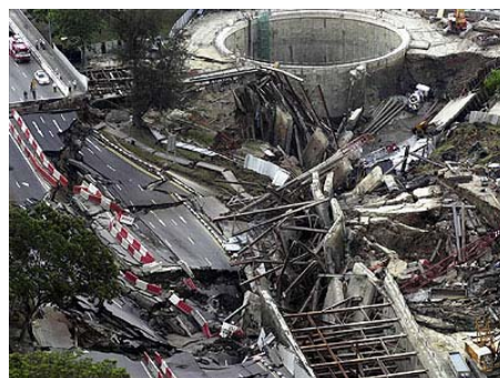
Failure of Nicoll Highway, Singapore (20 th April 2004)
